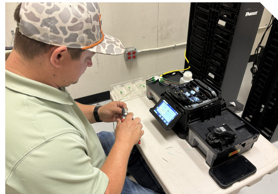
PHOTO: An ITS team member installs and updates campus technology to keep systems running smoothly. (FSU Network Communications and Technology)
