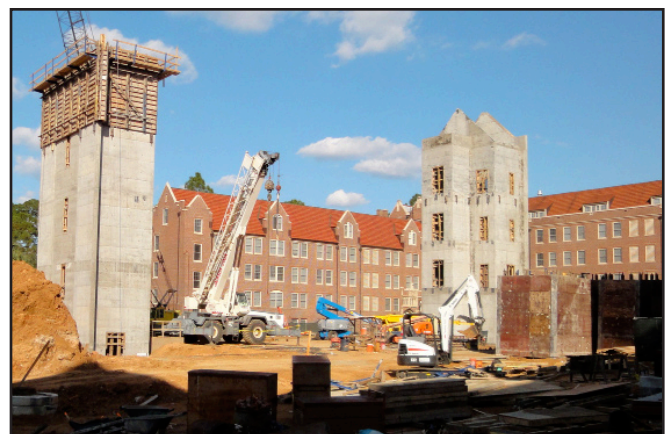
The staircases and elevator shafts of the HSF House are beginning to emerge.
